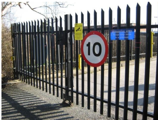
Figure 3 - Substation signage missing
