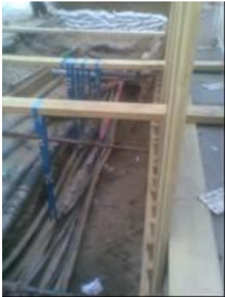
Figure 23: HV Cables exposed behind the fault
