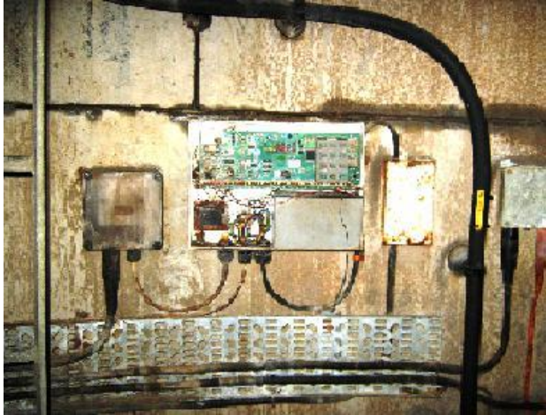
Figure 57: After effects of flooding on tunnel control equipment
