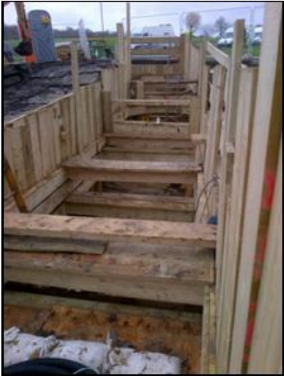
Figure 40: Berry Hill Joint Bay
