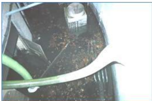
Figure 13: Flooded Substation at Bishops Bridge Road
