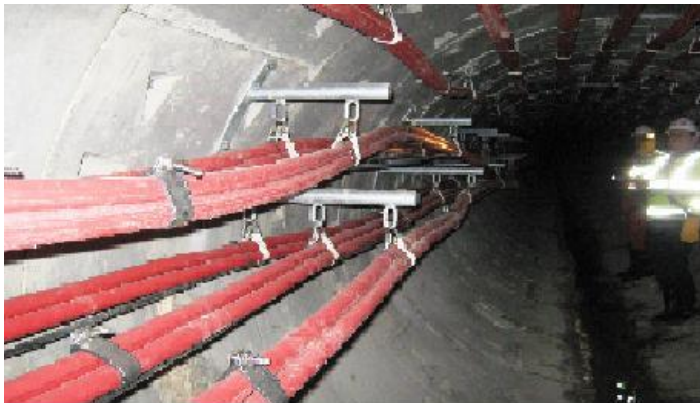
Figure 54: Movement of cables due to high ambient temperature
