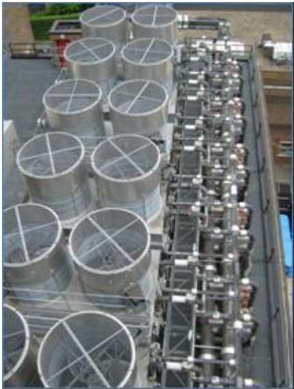
Figure 50: Cooling systems and pipework on the roof of Bankside Substation
