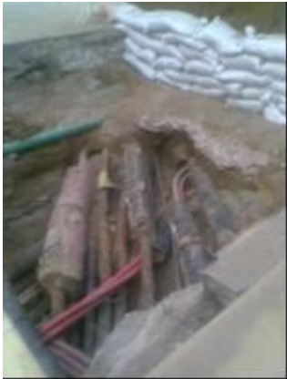
Figure 24: Cable congestion at the fault position
