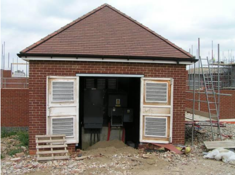
Figure 10: Substation in Suburban area with good access
