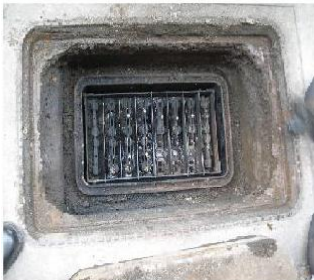
Figure 16: A Link box that has suffered a flashover due to a fault.
