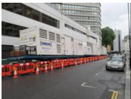
Figure 28: Penta Hotel - generation required for transformer change
