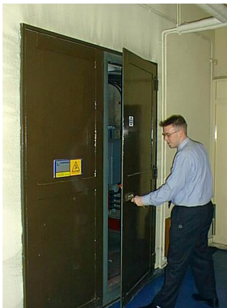
Figure 11: Restricted access Substation access at basement level
