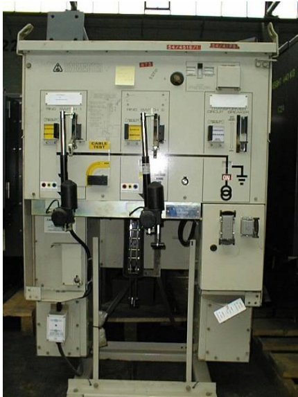
Figure 17: One of the items of HV switchgear that is "Trip tested"
