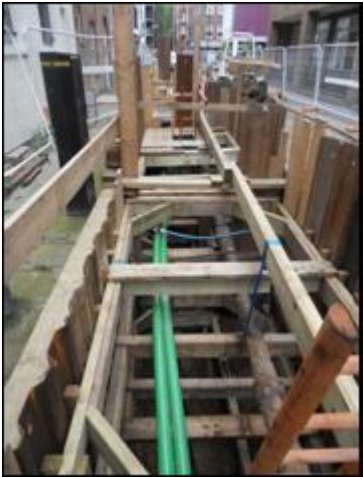
Figure 34: 7m deep Shaft to access Backhill to Fisher St Oil filled cable
