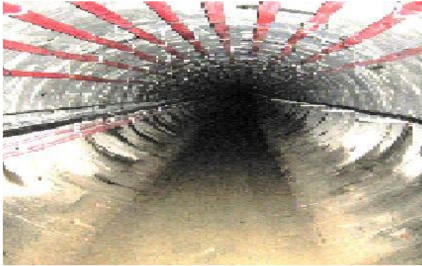
Figure 56: Millennium cable tunnel under the River Thames towards the flooding
