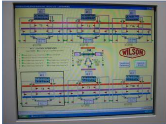
Figure 66: Heat recovery system control panel
