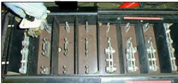
Figure 15: Serviceable link box with Links and a fuse being inserted
