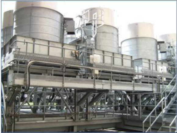
Figure 64: Cooling towers on the roof of Bankside Substation
