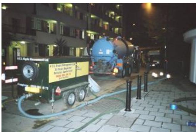
Figure 12: Tanker and Filter unit at Bishops Bridge Road flooded Substation
