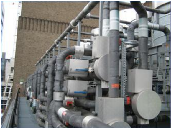
Figure 65: Valves and pipework for the heat recovery system
