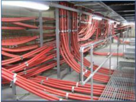
Figure 47: 11kV cables in a Substation cable basement
