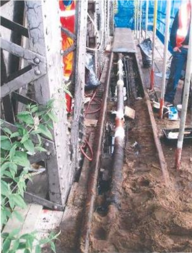
Figure 44: Leaking oil cable crossing Ranelagh Bridge
