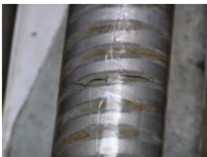
Figure 29: Lead sheath cracked on an oil filled cable
