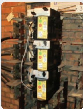
Prototype Circuit Breakers Installed to a distribution board in an IFI trial
