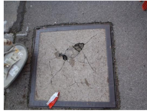
Figure 6: Poor condition cover
