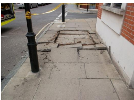
Figure 3: Footway disruption following a cable failure
