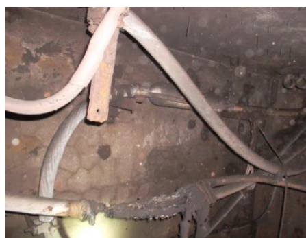
Figure 4: Status of the cable following failure
