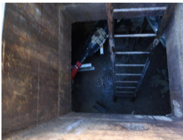
Figure 2: Example of a large cable pit with a number of cables and joints
