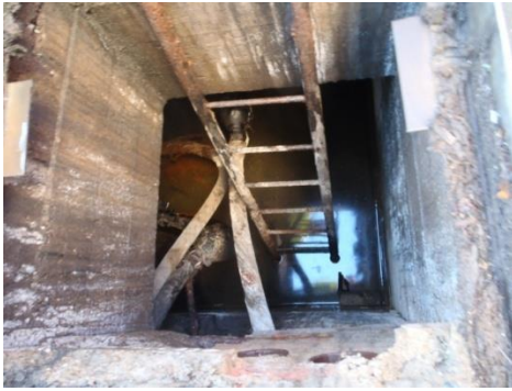
Figure 5: Poor condition ladder
