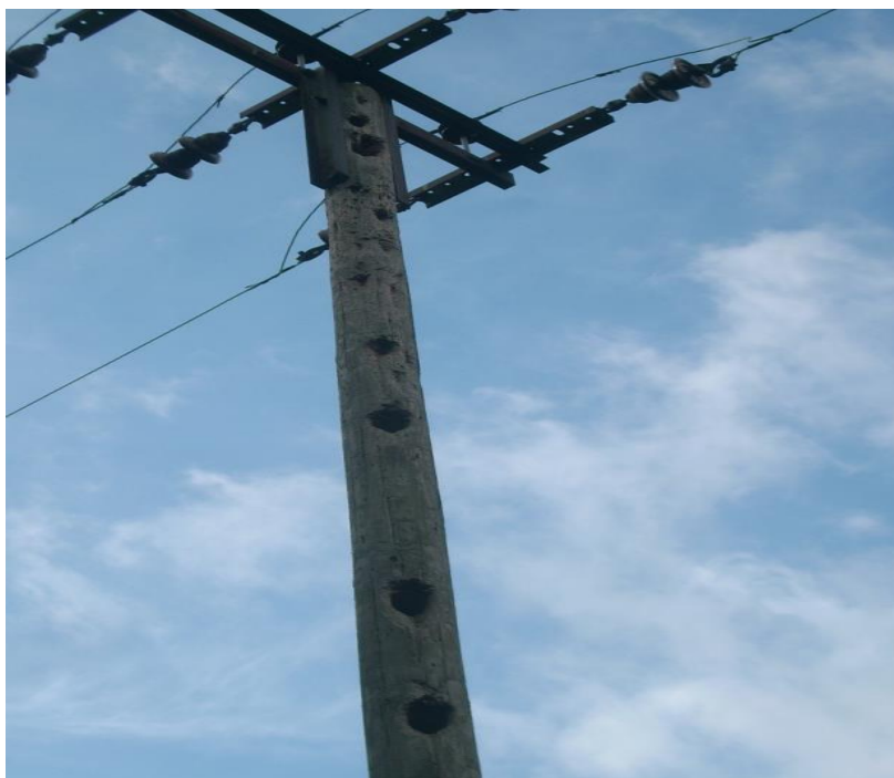
Figure 34 – Woodpecker damage on a HV wooden pole
