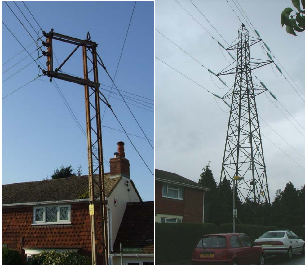
Figure 1 – a narrow-based (left) and broad-based (right) tower, side-by-side, illustrating the differences in design and construction
