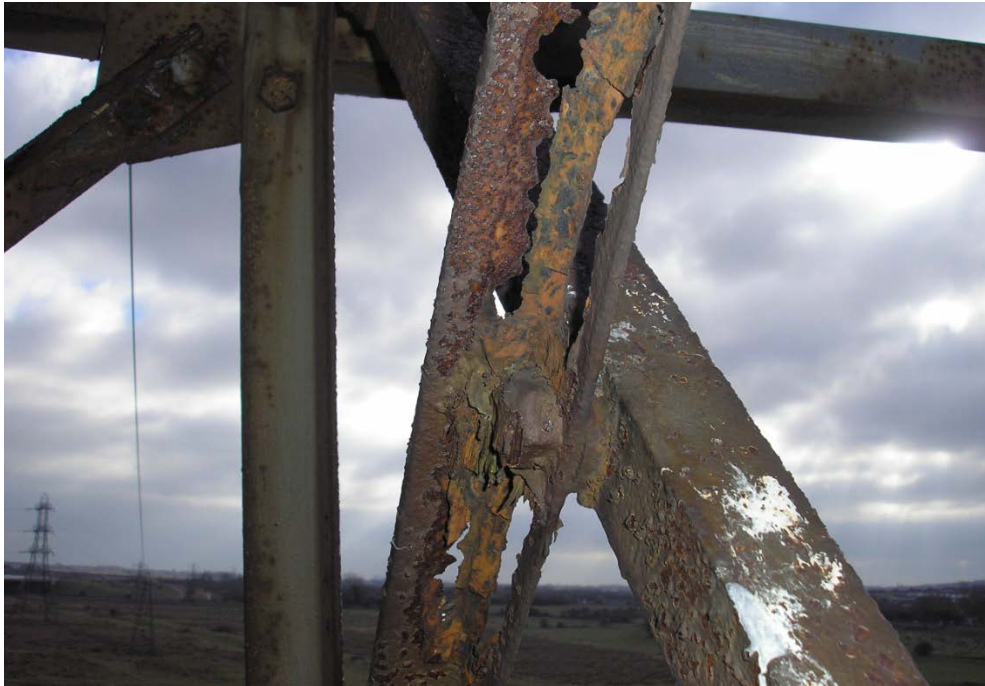
Figure 9 : A very poor condition tower steelwork member, illustrating the extremes of deterioration that can be found on the UK Power Networks assets
