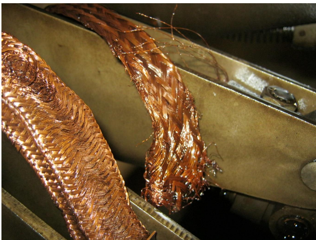
Figure 44 – Recording the condition of diverter braids in tap-changers improves our understanding of their wear and maintenance requirements
