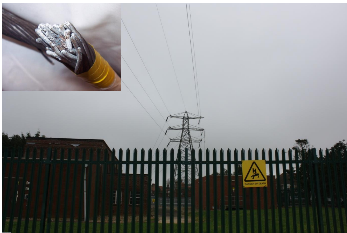
Figure 3 – Failed single phase span of 132kV conductor
