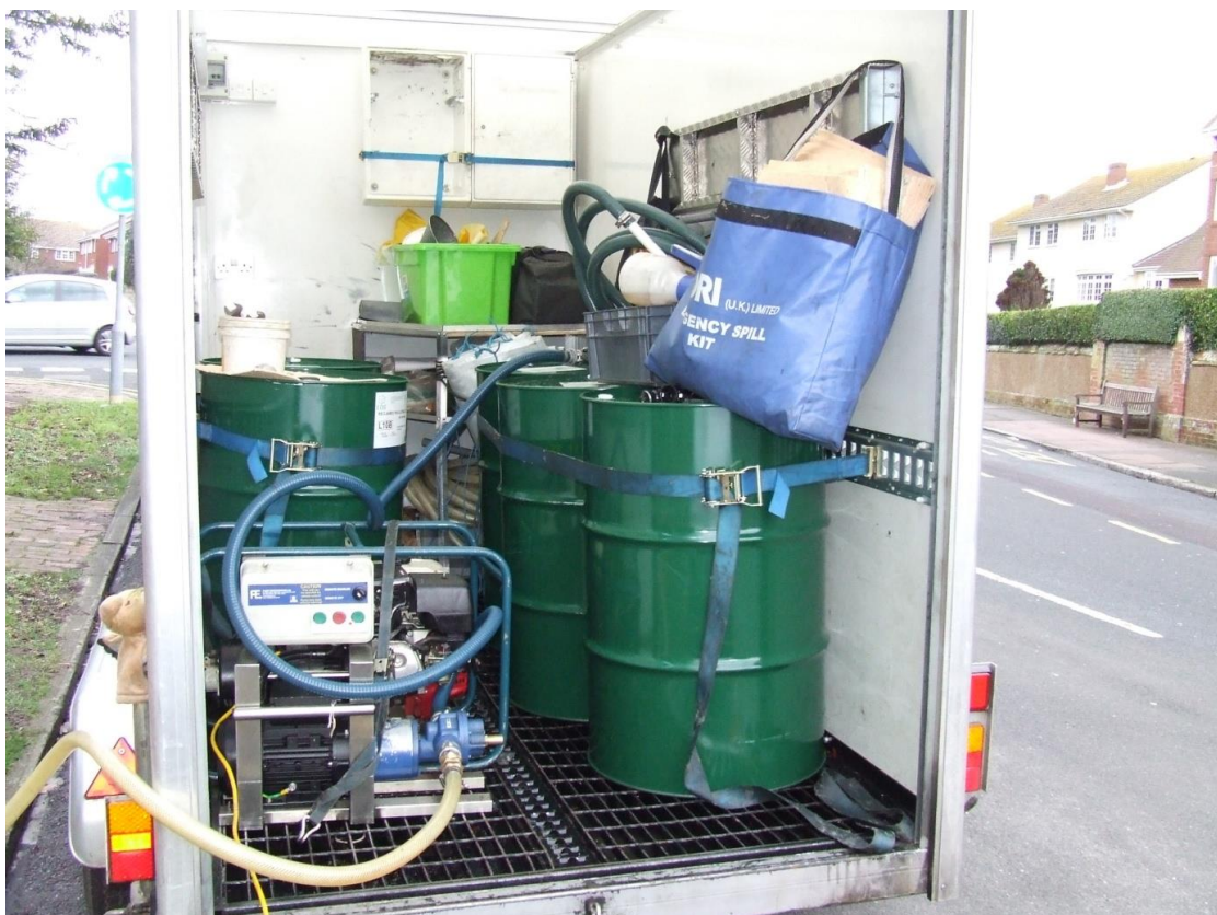
Figure 38 – Secondary substation maintenance oil-handling facilities
