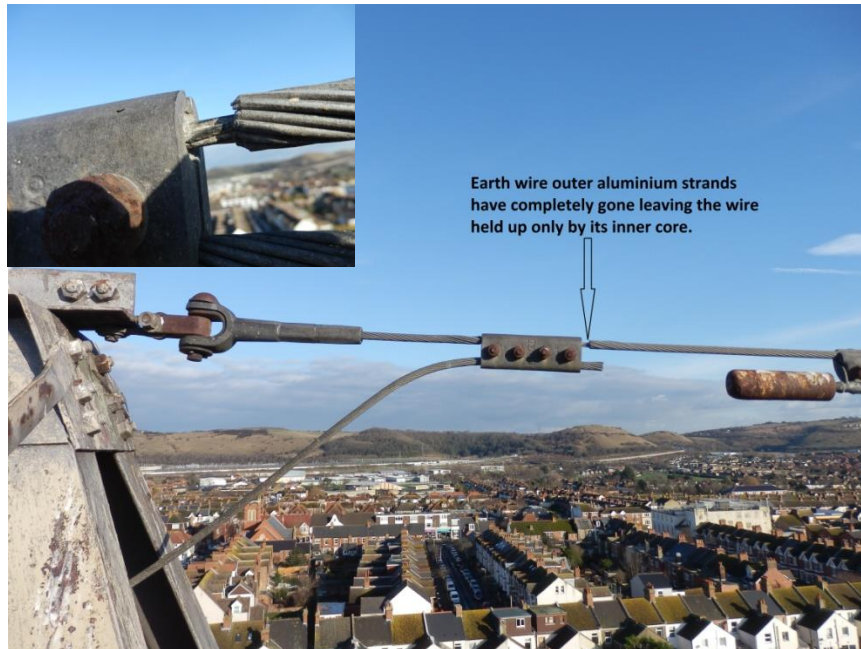
Figure 6 – Condition of conductor and fitting
