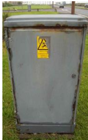
Figure 13: Corroded LV Network Pillar
