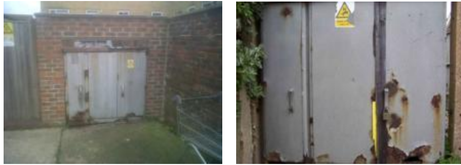
Figure 12: Badly Deteriorated LV Substation Pillar at Wilmot Road, Shoreham-By-Sea
