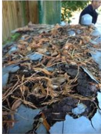
Figure 9: Severe Corrosion and Debris Accumulation
