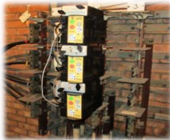
Figure 32: LV CBs installed on an LV board
