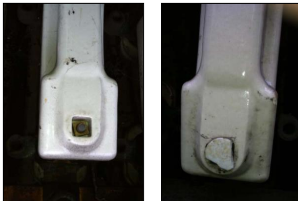
Figure 22: Damaged Fused Barriers
