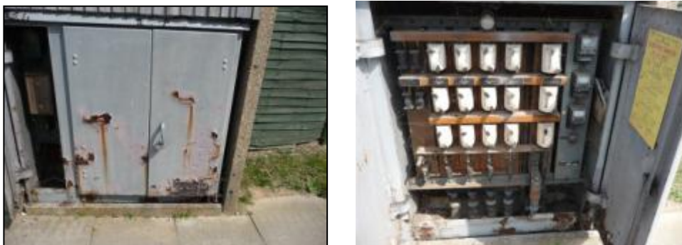
Figure 11: Badly Deteriorated LV Pillar at Cotswold Way, East Preston
