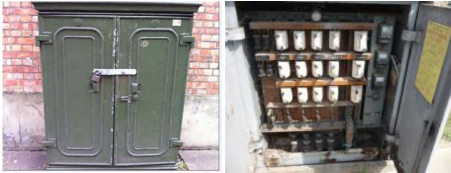
Figure 21: Defective Door and Damaged Fused Barriers
