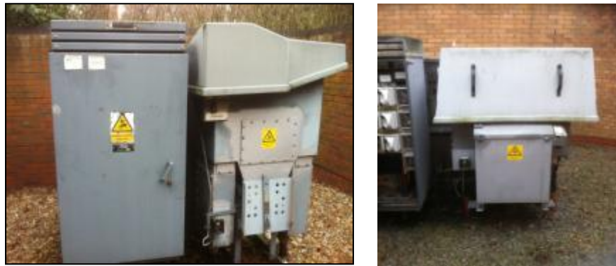
Figure 10: Weather covers fitted to a LCR T4GF3 RMU and a LUC FRMU2A RMU
