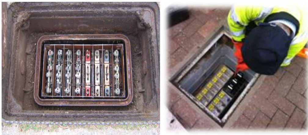
Figure 33: Before and after: Switches Installed to a LB in place of Standard Links
