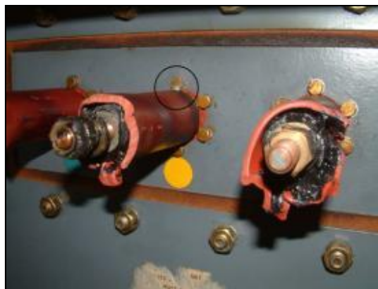
Figure 18: White Deposits on Yellow Phase Bushing Bolts
