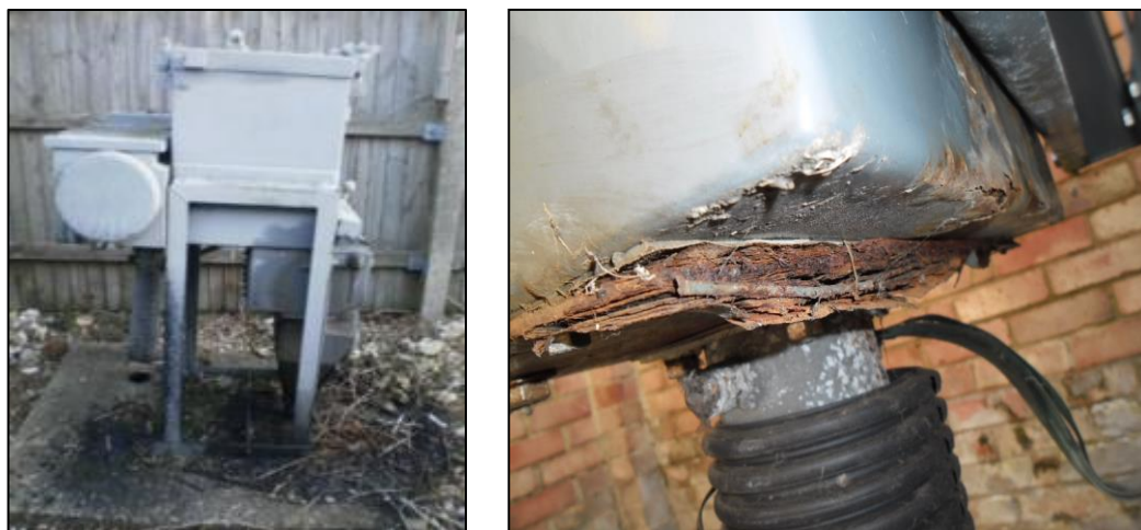
Figure 16: Severe Oil-leak of a LCR ETV2 Switch Fuse at Lyndhurst Av, Rainham and a Defective Cable Box at Rowena Road, Westgate-on-Sea
