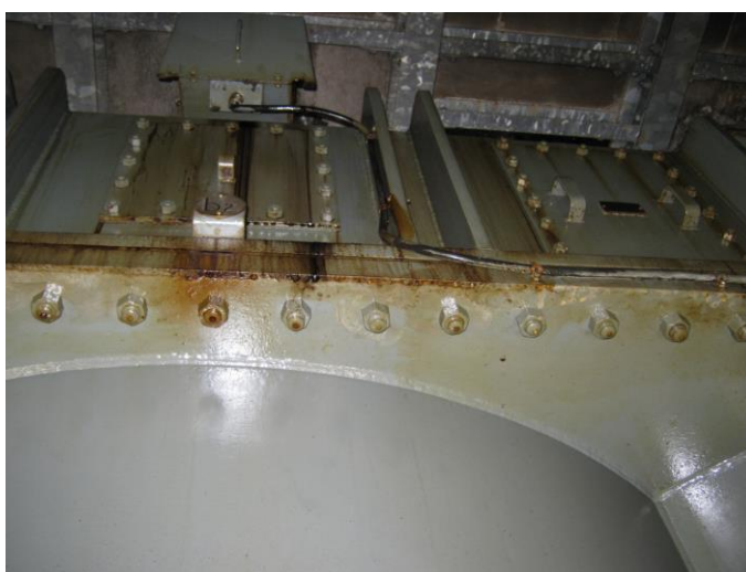
Figure 5 – Severe oil leak from main cover gasket, Chessington Grid GT2
