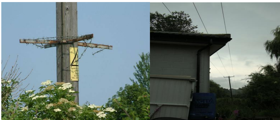
Figure 7– Defective anti-climbing device; Figure 8 -Ground Clearance highest priority, P5 priority is P3 or P4 depending on the ESQCR risk rating
