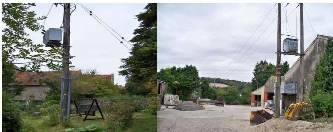
Figure 13- A pole transformer in a recreational area is a key risk requiring mitigation. Figure 14 -A pole transformer with evidence of farm machinery is a key risk requiring mitigation
