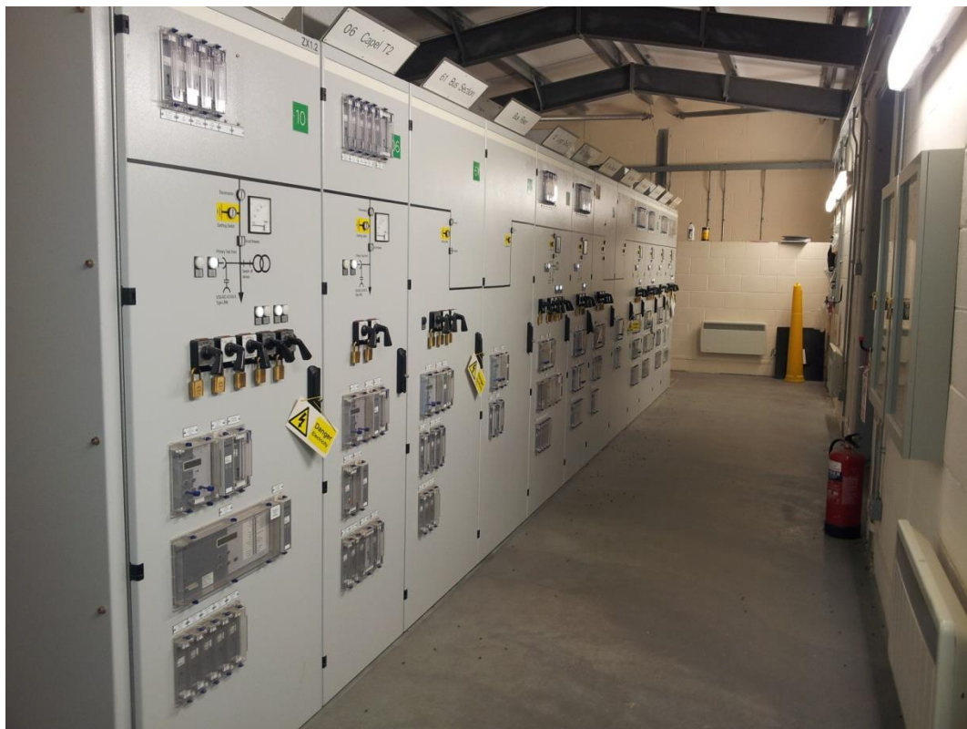
Figure 10 – ABB ZX1.2 switchboard
