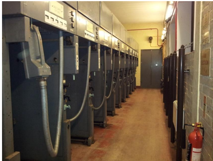
Figure 2 – Reyrolle L42T switchboard
