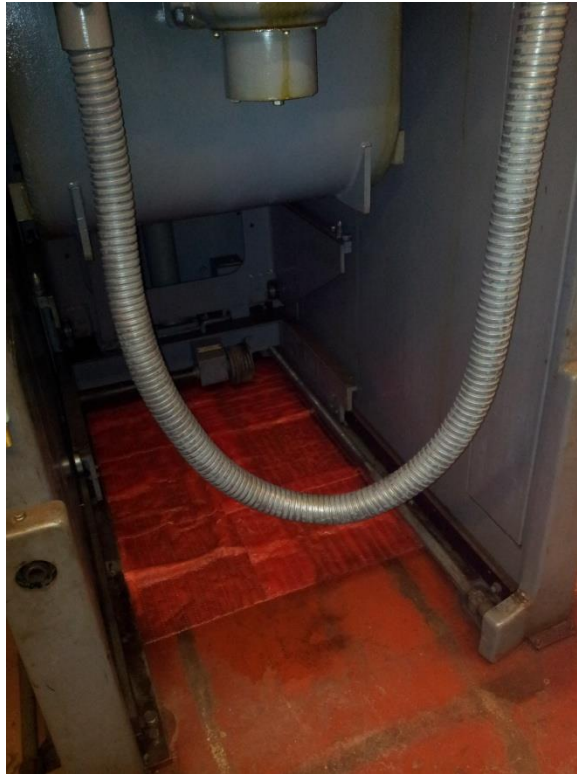
Figure 4 – Reyrolle L42T Oil Leak
