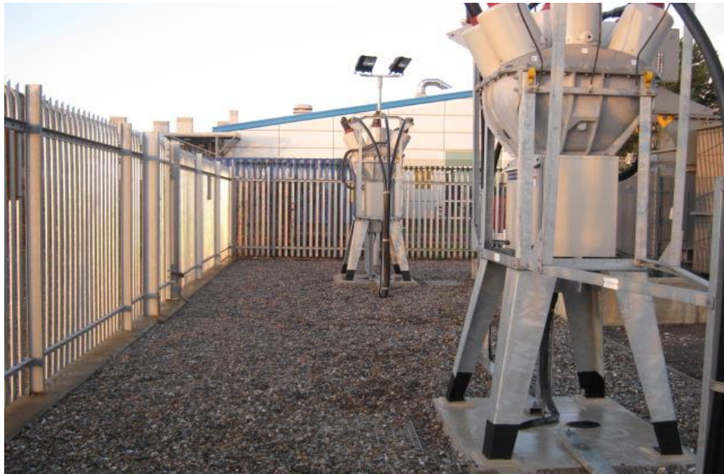
Figure 9 – Hawker Siddeley Switchgear Horizon
