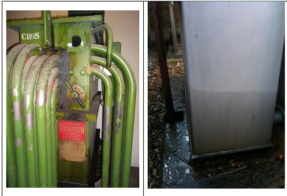
Figure 7 - Transformers in poor condition
