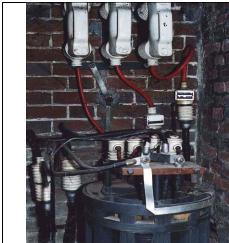
Figure 4: Typical 2kV s/s in a brick “lean-to” on customer’s house. LV fuse is on the left out of view. The porcelain caps on the air cooled transformer cover the tapping connections
