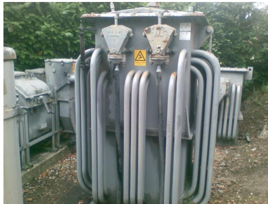
Figure 3 – Example of a Scott Transformer at Groombridge substation
