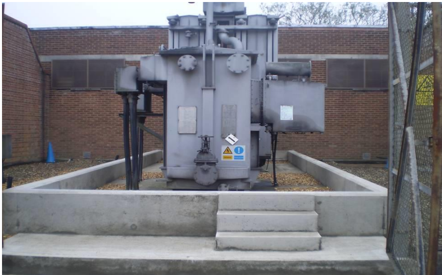
Sundon 11kV primary substation bunding
