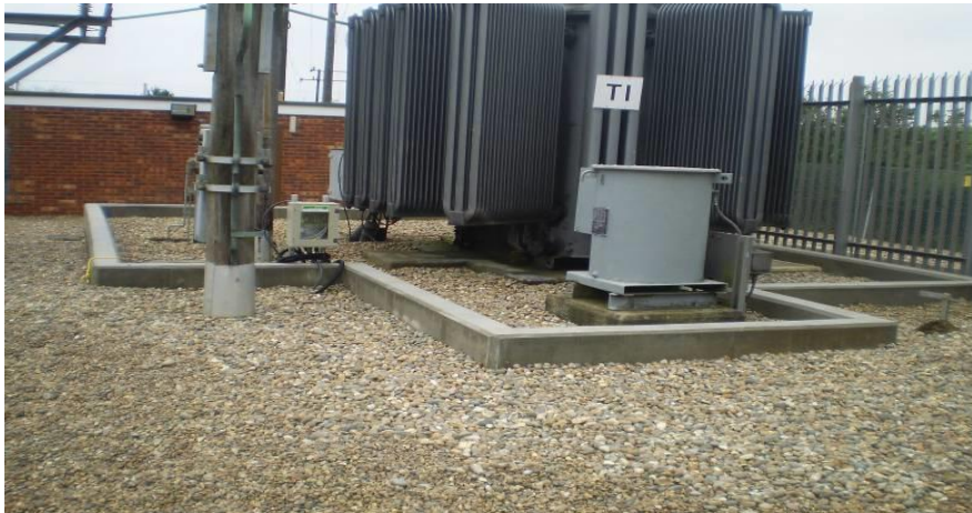
Rydon primary substation bunding
