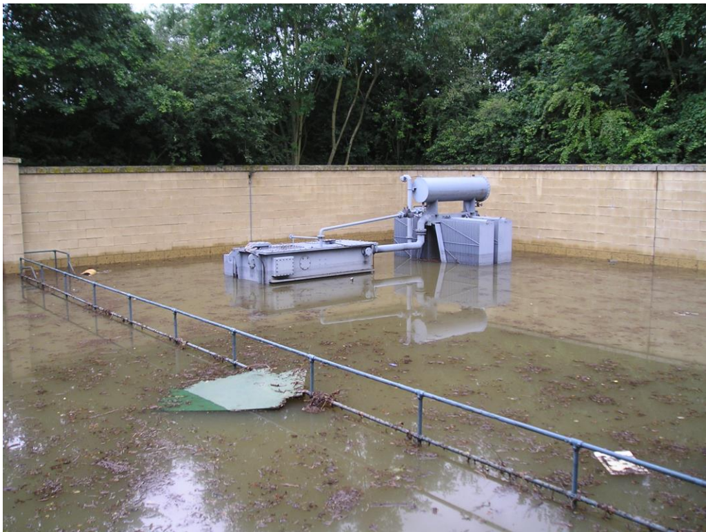
Figure 2 Example of flooded UK Power Network Substation
