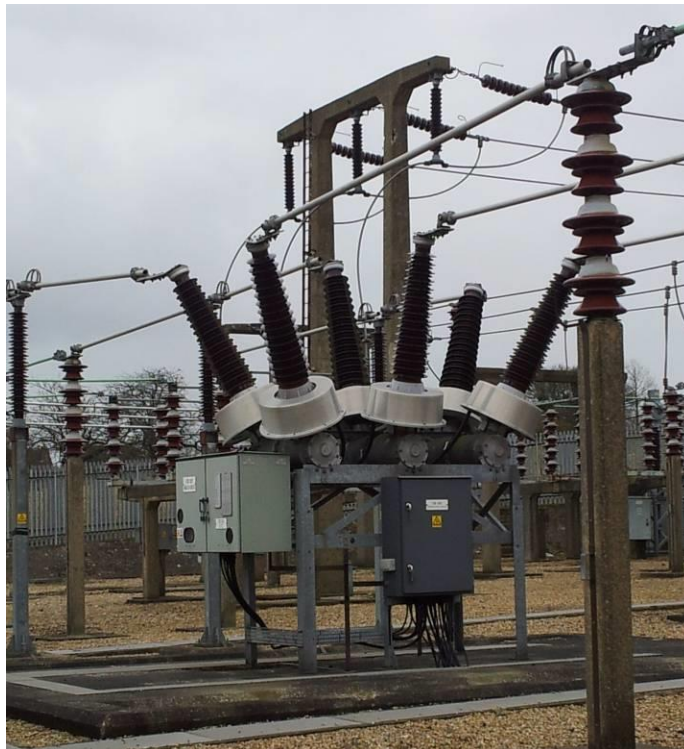
Figure 7 – Siemens 3AP1DT circuit breaker
