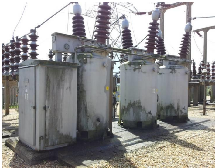
Figure 2 – GEC OFA11 bulk oil circuit breaker
