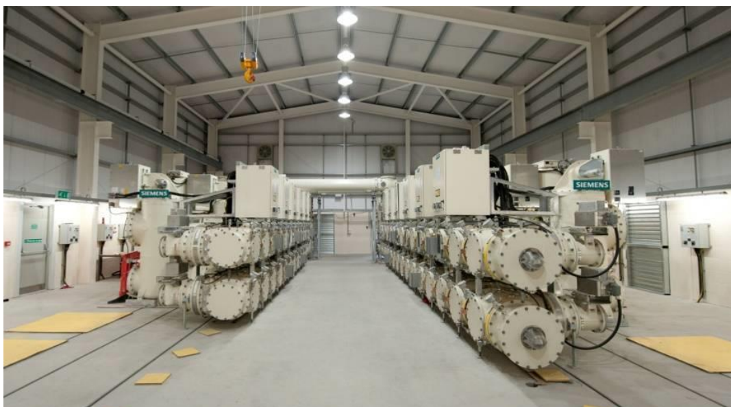
Figure 8 – Siemens 8DN8 GIS circuit breaker
