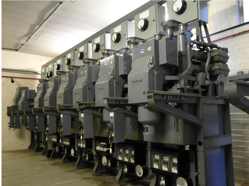
Figure 2 – Reyrolle ‘C’ switchgear at Addington Local substation
