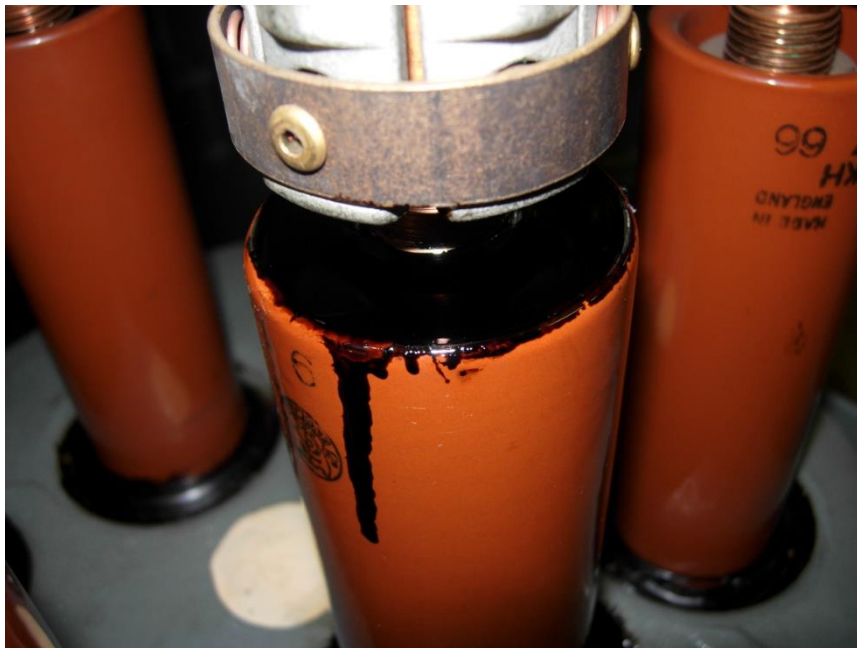
Figure 5 – Compound leak from C4X bushing at Moulescoombe substation
