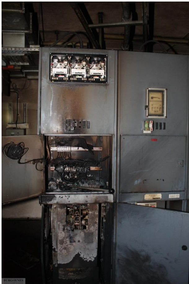
Figure 20 – GEC VMX: Failed 11kV panel
