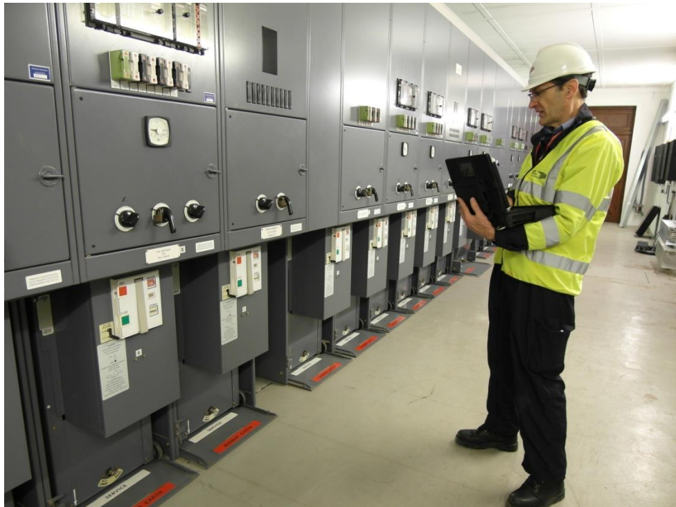
Figure 7 – Substation inspector with handheld device
