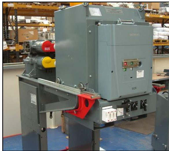
Figure 23 – Siemens Sion-C retrofit CB
