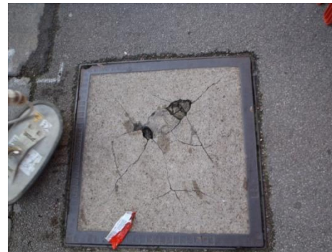
Figure 6: Poor condition cover
