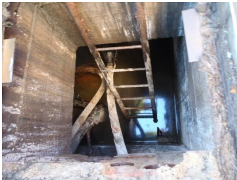
Figure 5: Poor condition ladder
