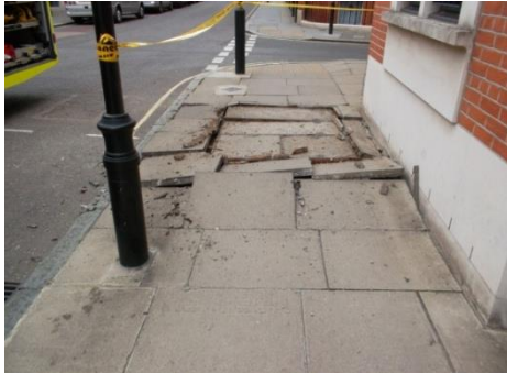
Figure 3: Footway disruption following a cable failure
