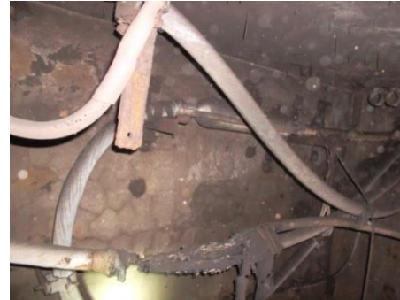
Figure 4: Status of the cable following failure
