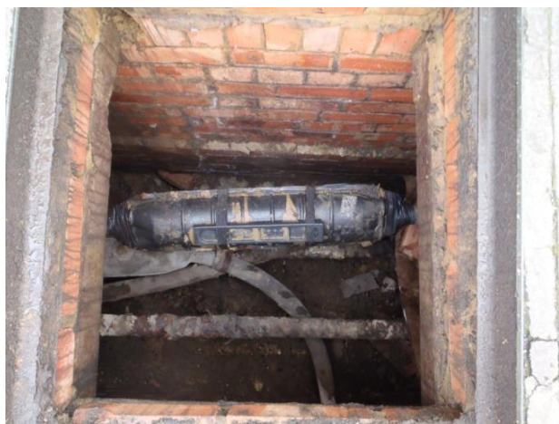
Figure 2: Example of a large cable pit with a number of cables and joints
