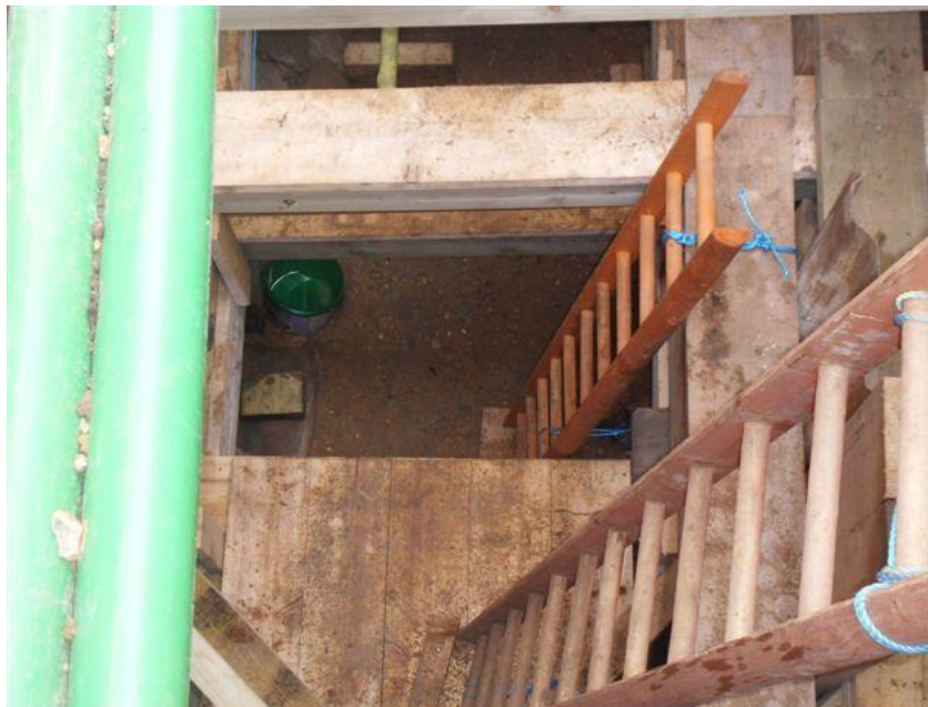
Figure 74 – The excavation was 7 metres deep (23 feet) below the ground and required a significant excavation
