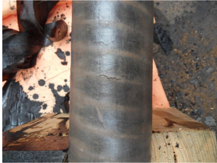
Figure 75 – The lead sheath was found to be crystallised
