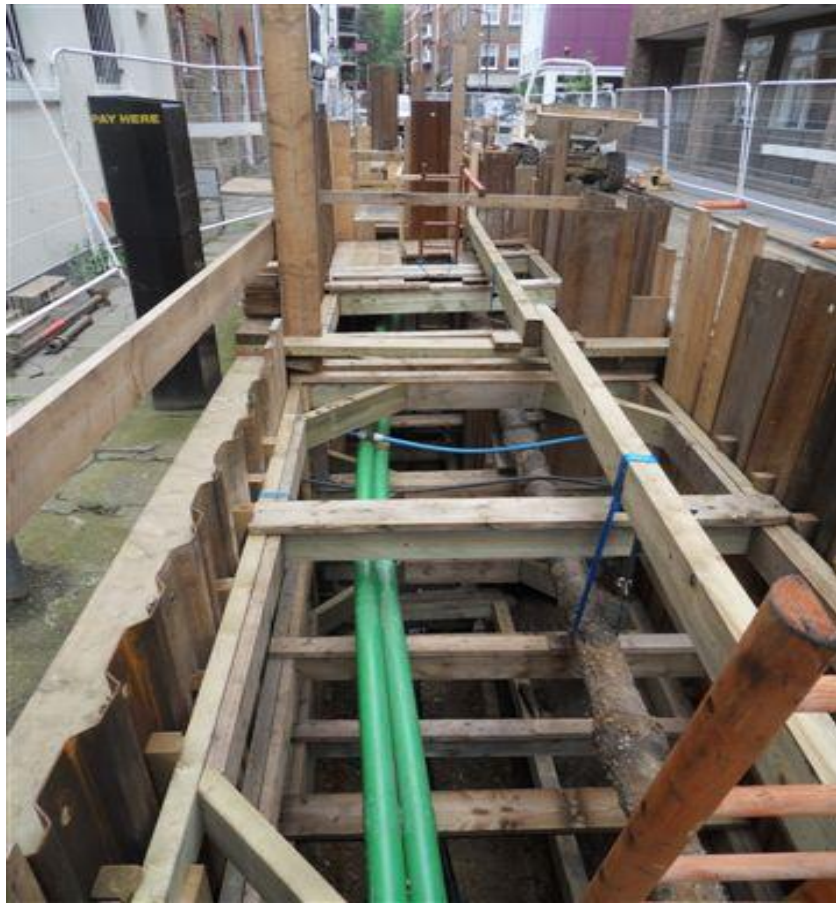
Figure 73 – Excavation required for fluid-filled cable repair at the Back Hill Fisher Street No 4 circuit
