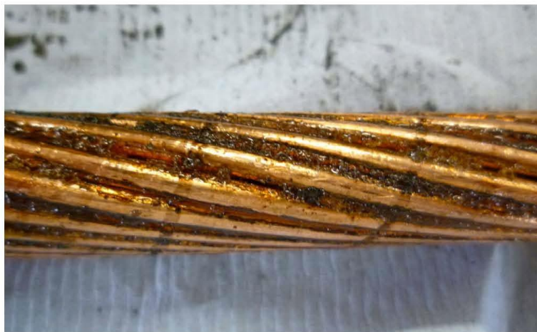
Figure 6: Hardened cable compound on conductors
