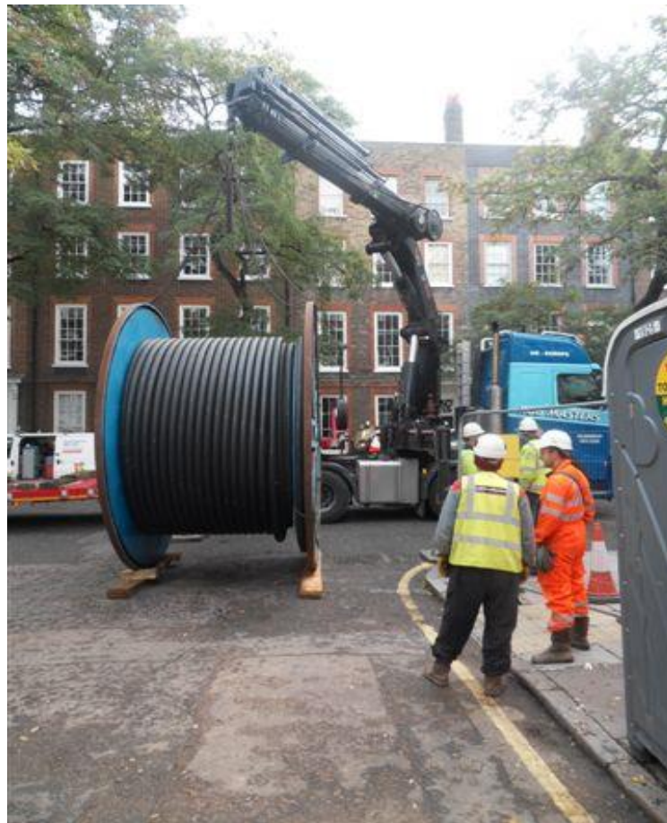
Figure 76 – The replacement fluid-filled cable is delivered to site by a specialist contractor
