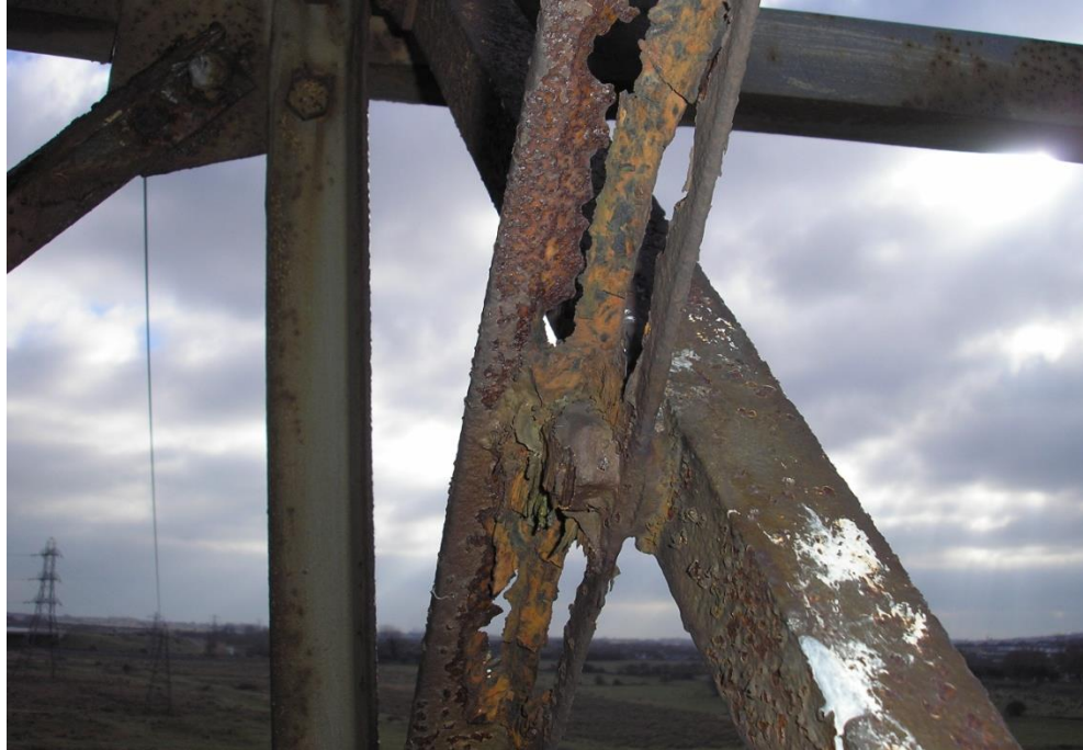
Figure 5: A very poor condition tower steelwork member, illustrating the extremes of deterioration that can be found on UK Power Networks assets
