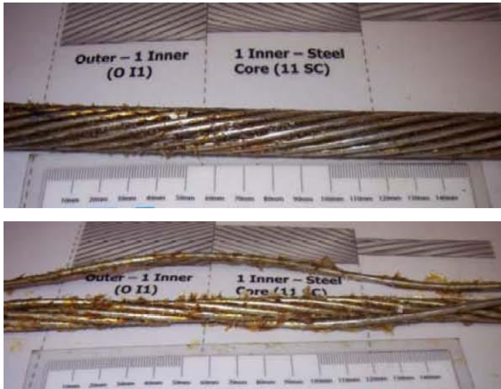
Figure 9: A poor condition ACSR conductor from an LPN route showing the extent of hidden corrosion that can occur between conductor strands
