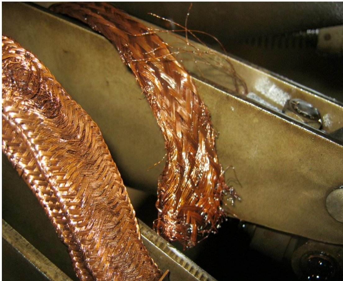
Figure 28 – Recording the condition of diverter braids in tap changers improves how we understand wear and maintenance requirements
