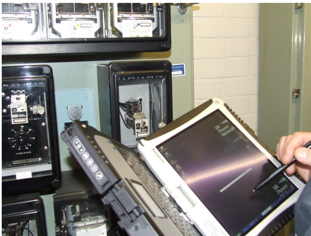
Figure 32 – Recording equipment condition on a portable device for automatic updating of the asset register
