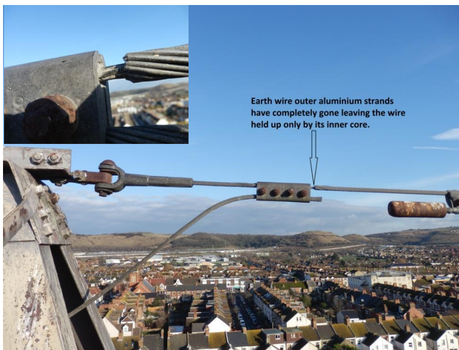
Figure 2 – Condition of conductor and fitting
