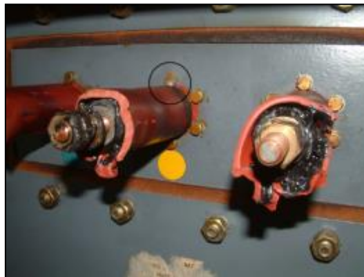
Figure 15: White Deposits on Yellow Phase Bushing Bolts
