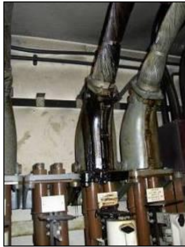
Figure 18: Leaking Top Entry Box at Park Lane
