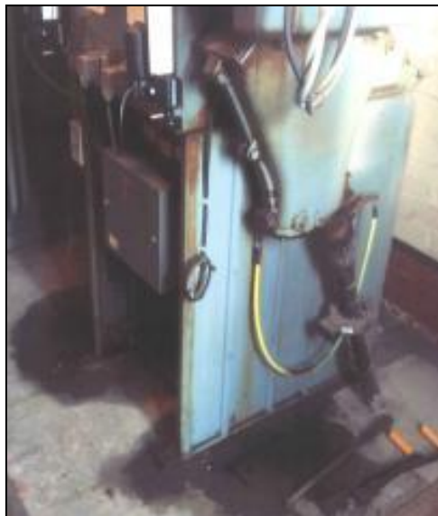
Figure 13: Severe RMU Oil Leak
