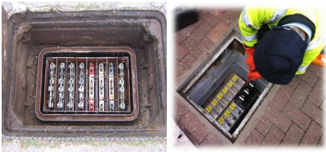
Figure 30: Before and After: Switches Installed to a LB in place of Standard Links
