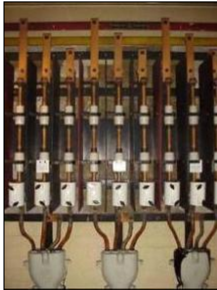
Figure 10: Cornwall Gdns 5 Substation
