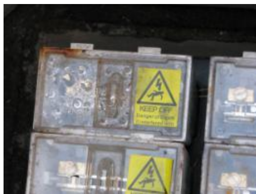
Figure 20: Water Ingress caused by Condensation
