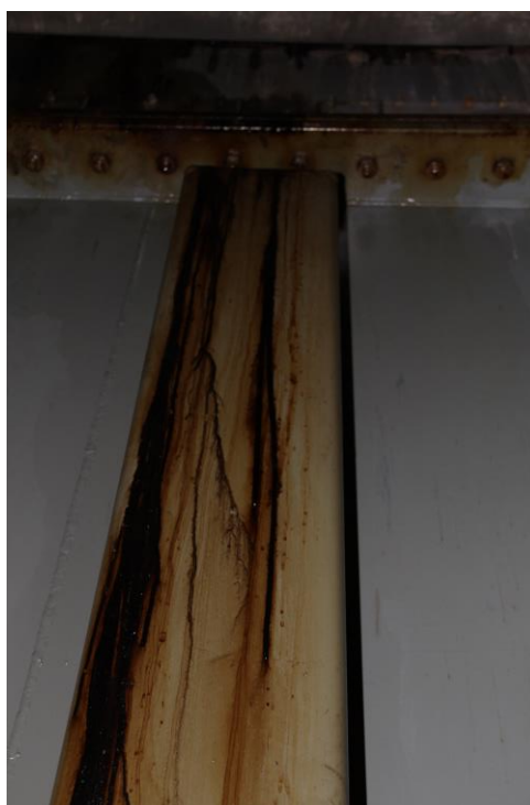
Figure 5 – Severe oil leak from main cover gasket, Bengeworth Road GT2
