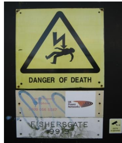
Figure 2 - Vandalised Sign with graffiti
