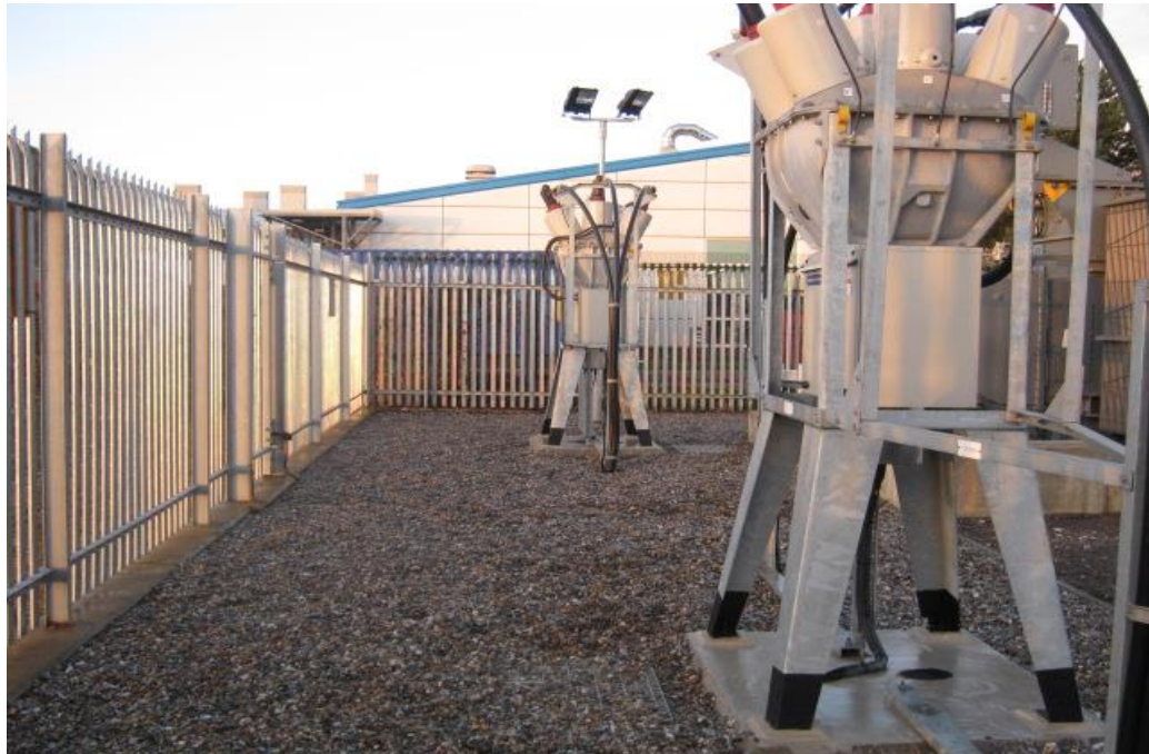
Figure 8 – Hawker Siddeley Switchgear Horizon
