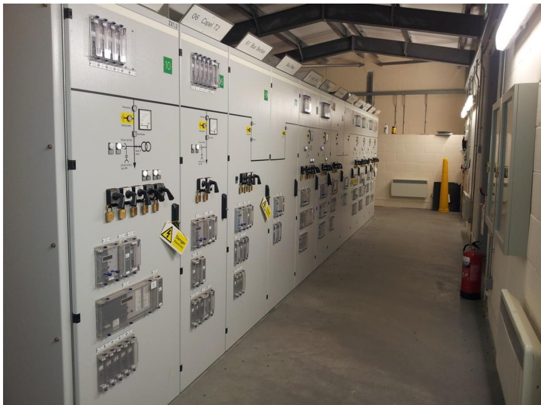
Figure 9 – ABB ZX1.2 switchboard
