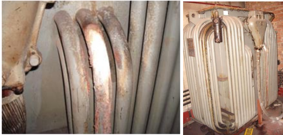
Figure 3 - Transformers in poor condition at Queenhithe Hotel, Paternoster
