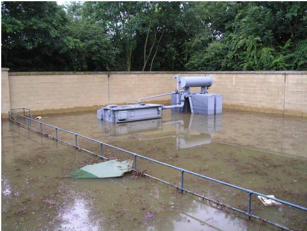
Figure 2 Example of flooded UK Power Network Substation
