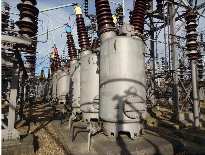
Figure 3 – AEI OW circuit breaker
