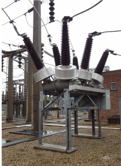
Figure 9 – Siemens 3AP1DT circuit breaker
