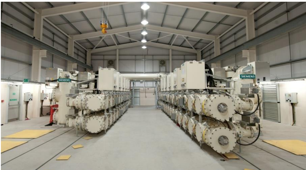
Figure 10 – Siemens 8DN8 GIS circuit breaker
