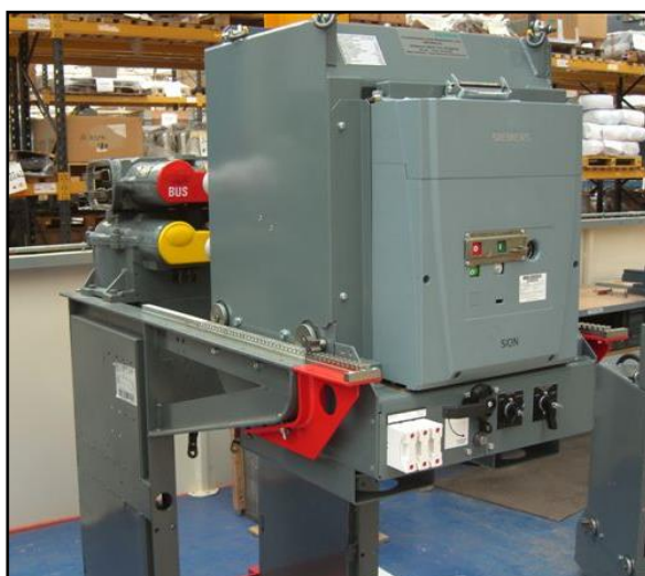
Figure 21 – Siemens Sion-C Retrofit CB
