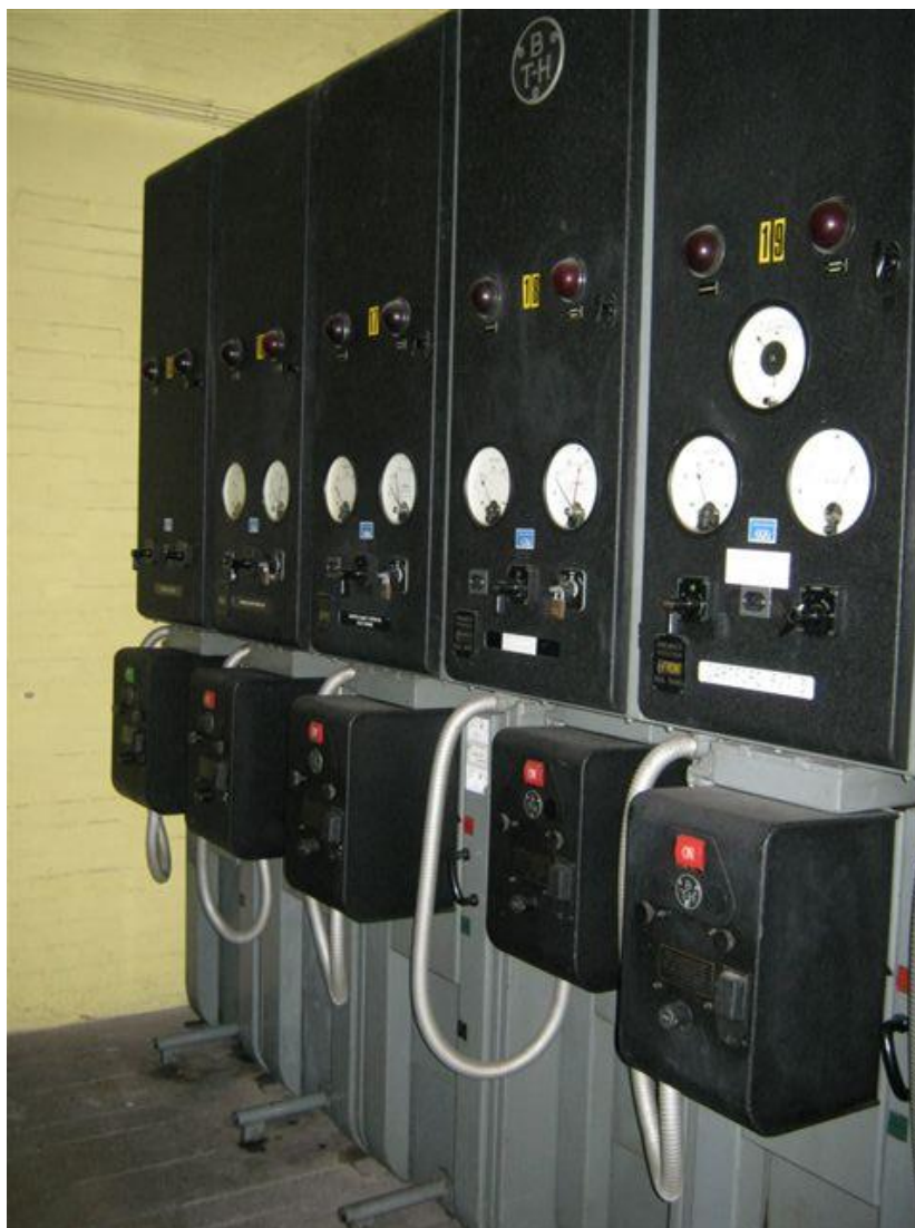
Figure 2 – BTH 'QF' switchgear at Clapham Park Rd substation
