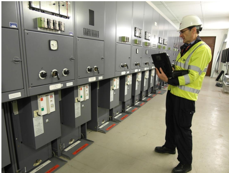
Figure 8 – Substation inspector with handheld device
