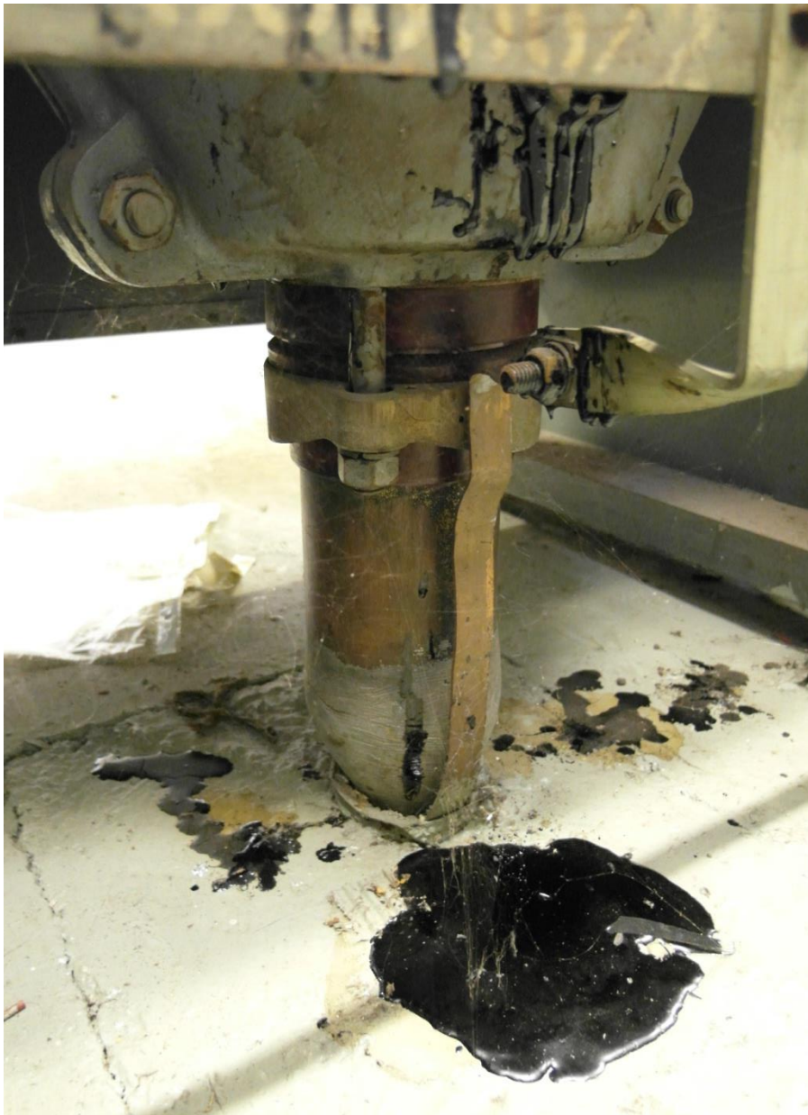
Figure 7 – Typical compound leak from a cable box
