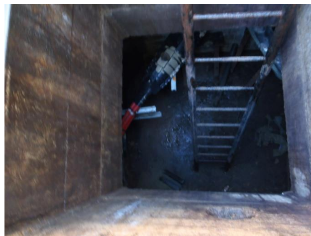
Figure 2: Example of a large cable pit with a number of cables and joints
