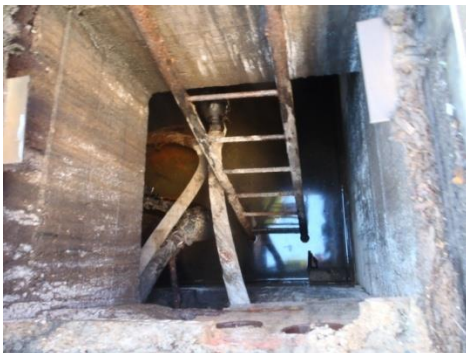
Figure 5: Poor condition ladder
