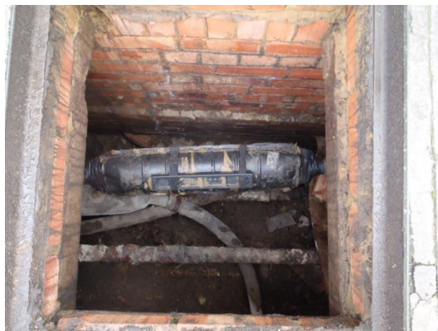
Figure 1: Example of a small cable (<1m 3 ) pit with service joint
