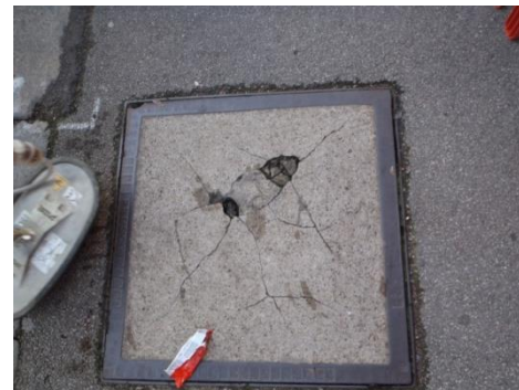
Figure 6: Poor condition cover
