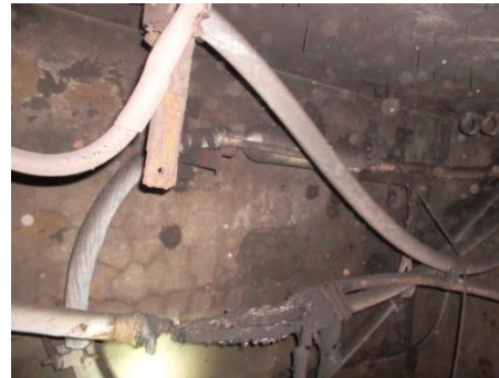
Figure 4: Status of the cable following failure
