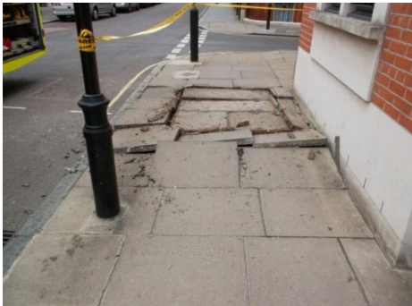
Figure 3: Footway disruption following a cable failure
