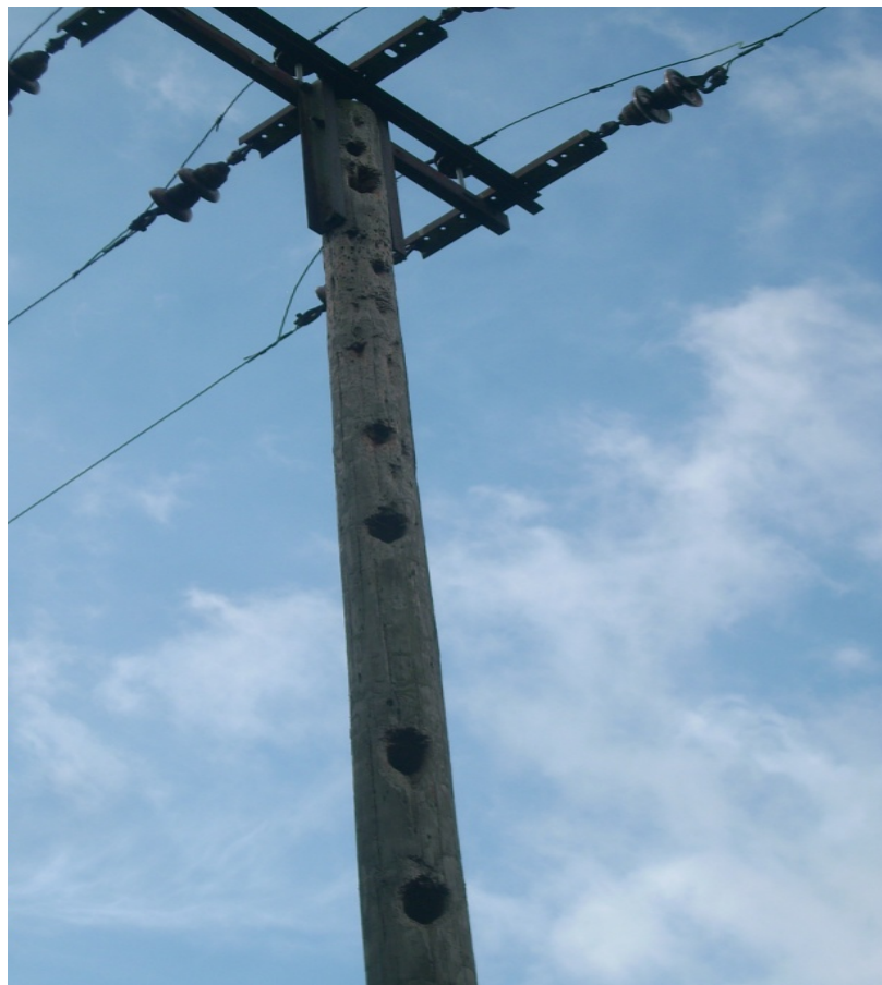
Figure 35 – Woodpecker damage on an HV wood pole
