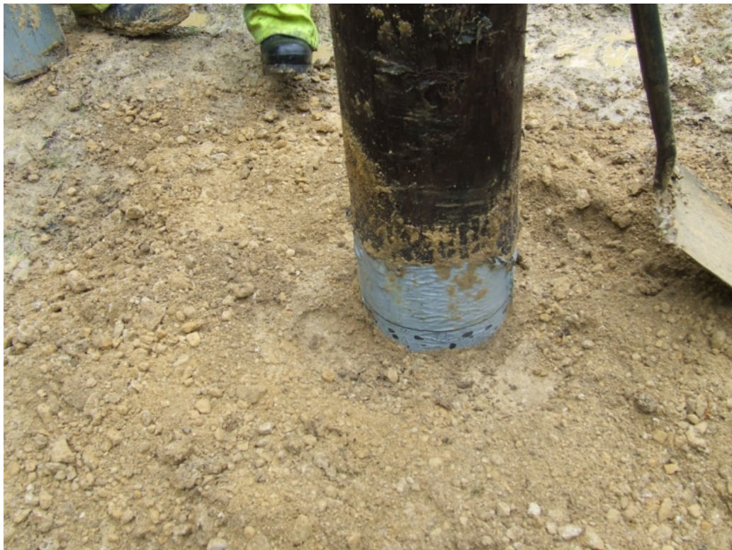
Figure 32 – Pole saver installed on a wood pole
