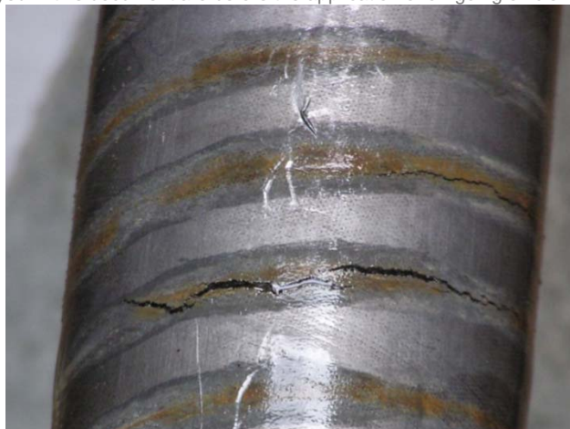
Figure 13 – Crystallised lead sheath
