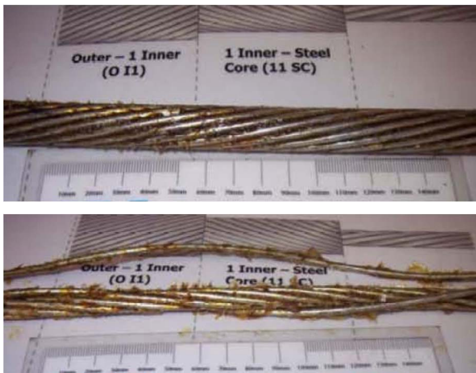
Figure 13: A poor condition ACSR showing the extent of hidden corrosion that can occur between conductor strands
