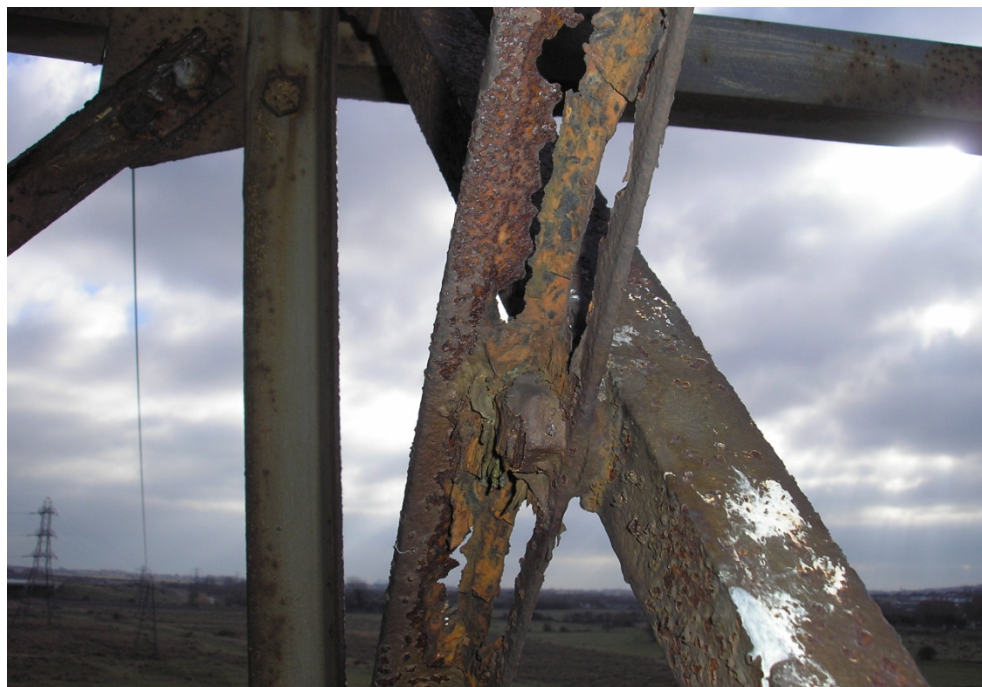
Figure 9: A very poor condition tower steelwork member, illustrating the extremes of deterioration that can be found on UK Power Networks assets
