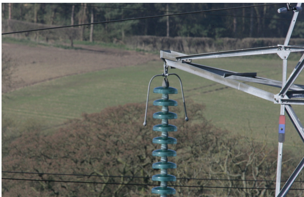
Figure 11: An enlarged portion of an EPN tower on Route PPA, showing the level of detail of a condition appraisal that can be carried out from a desktop assessment
