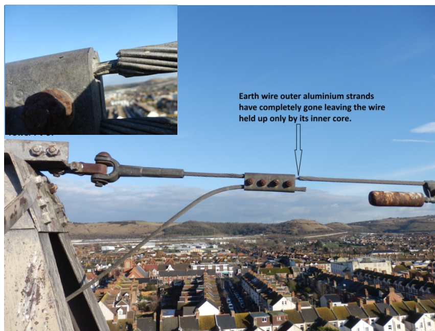
Figure 5 - Condition of Conductor and Fitting
