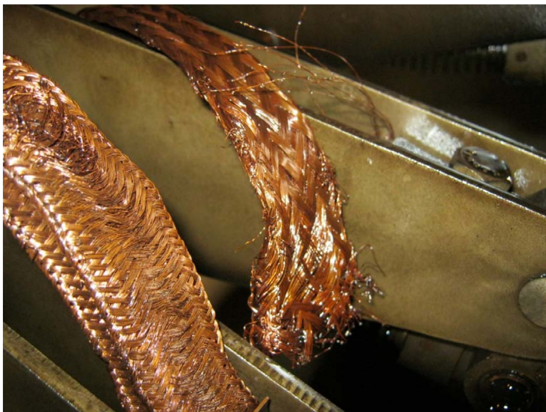
Figure 41 - Recording the condition of diverter braids in tap changers improves how we understand wear and maintenance requirements
