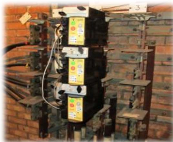
Figure 31: LV CBs installed on an LV board
