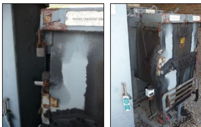
Figure 14: Severe Oil Leak (Yorkshire TYKE RMU)
