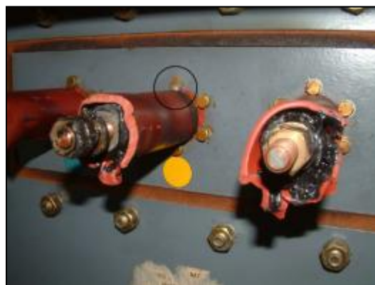
Figure 16: White Deposits on Yellow Phase Bushing Bolts
