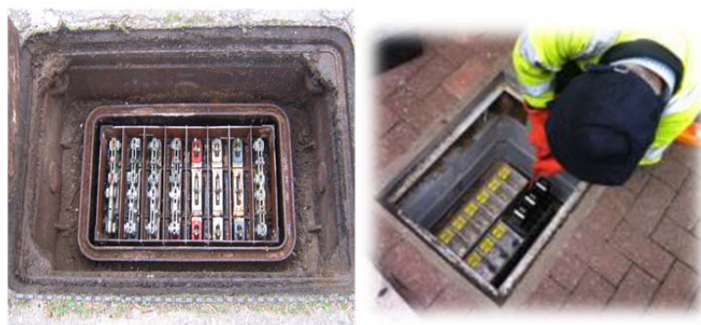
Figure 32: Before and After: Switches Installed to a LB in place of Standard Links
