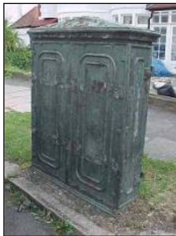
Figure 10: Badly Deteriorated LV Pillars
