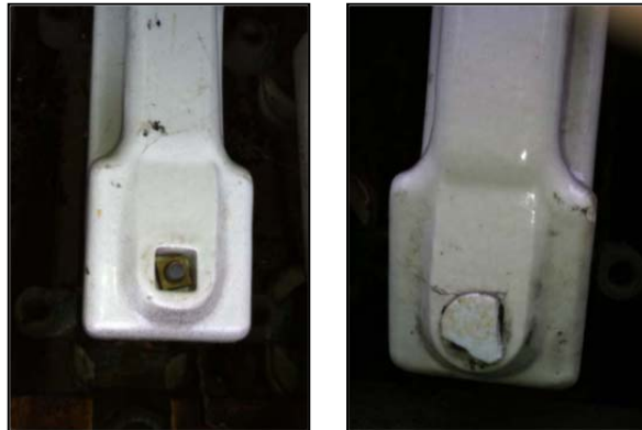
Figure 20: Damaged Fused Barriers
