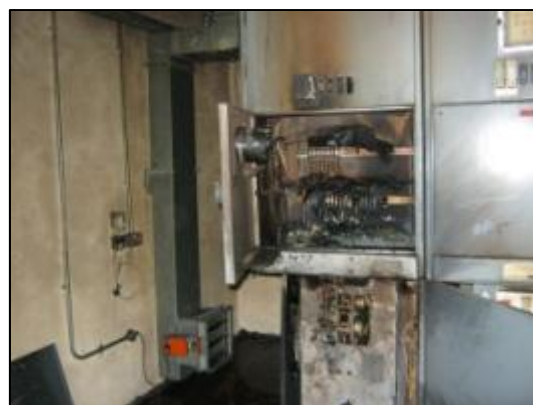
Figure 17: Failure of GEC VMX CB due to Partial Discharge
