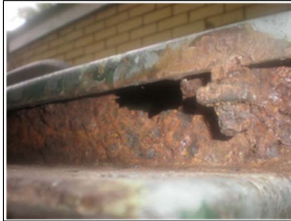
Figure 9: Severely Corroded BRU HFE Oil Switch Fuse Astons Road, Moor Park
