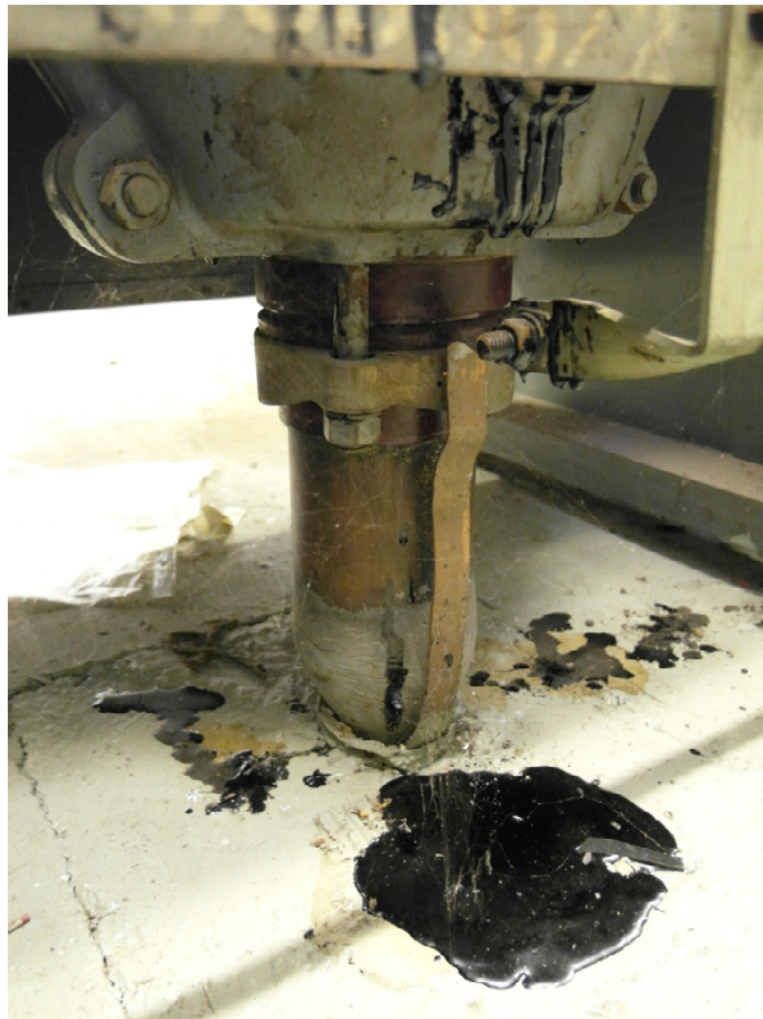
Figure 7 Typical compound leak from a cable box
