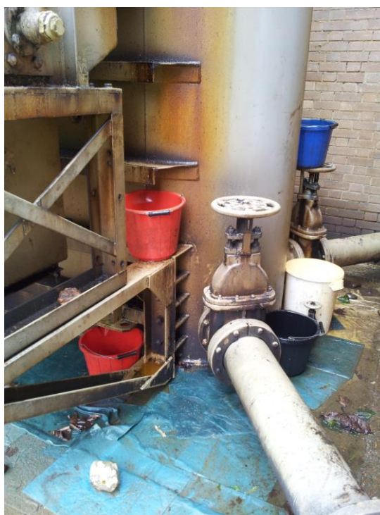
Figure 5 – Severe oil leak from main cover gasket, Kenton Primary T2
