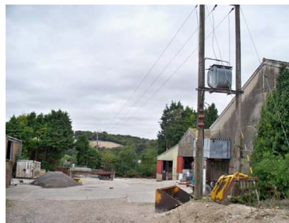
Figure 14 – A pole transformer with evidence of farm machinery is a key risk requiring mitigation
