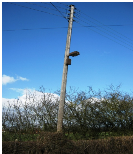
Figure 1 – Signage missing/fallen off
