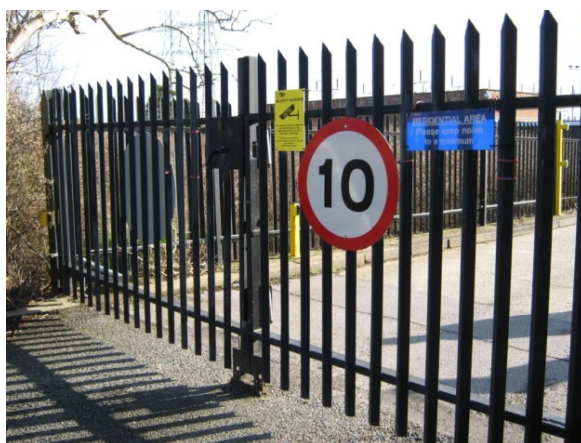
Figure 5 – Substation signage missing
