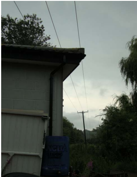
Figure 8 – Building clearance issue
