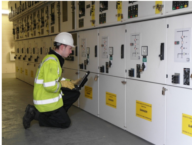
Figure 8 – Substation inspector with handheld device
