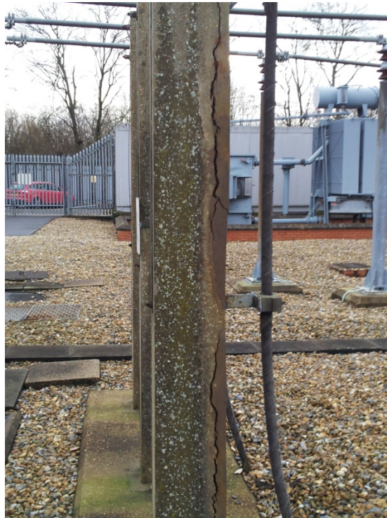
Figure 2 – Poor-condition support structure
