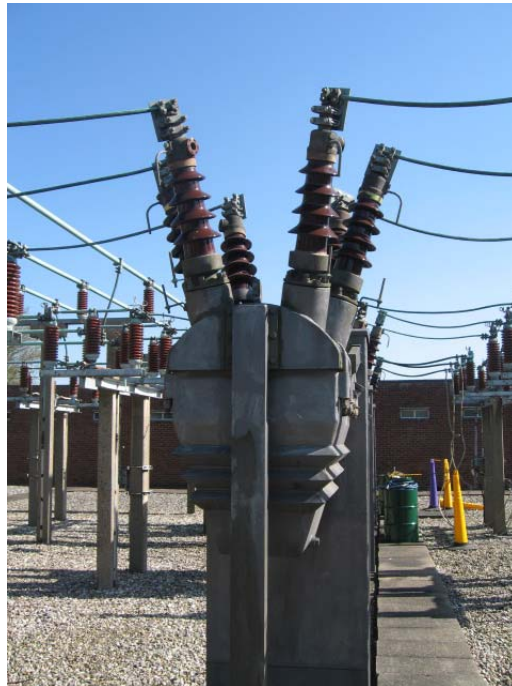
Figure 3 – Switchgear and Cowans K30 circuit breaker
