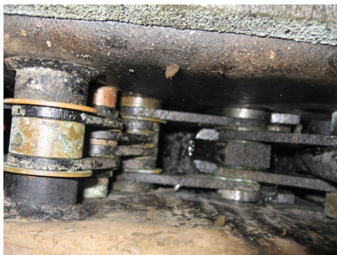
Figure 4 – Switchgear and Cowans K30 mechanism
