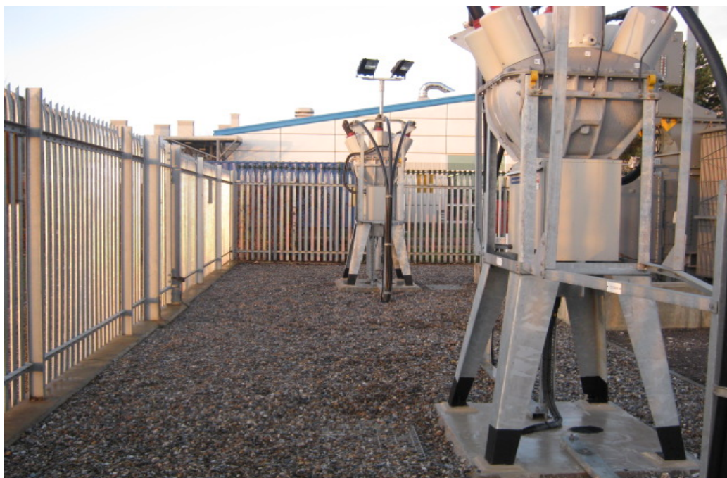
Figure 9 – Hawker Siddeley Switchgear Horizon
