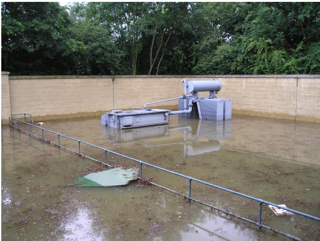
Figure 2 Example of flooded substation in UK Power Network Substation
