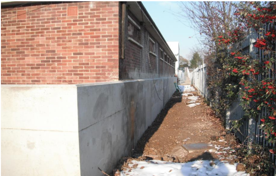
Flood alleviation wall constructed of concrete/steel around relay room
