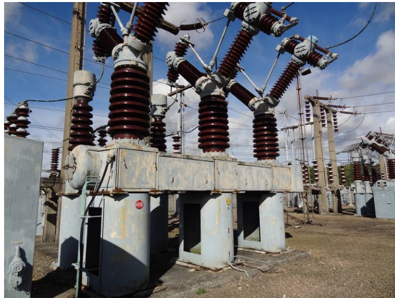
Figure 2 – Reyrolle OBYR circuit breaker
