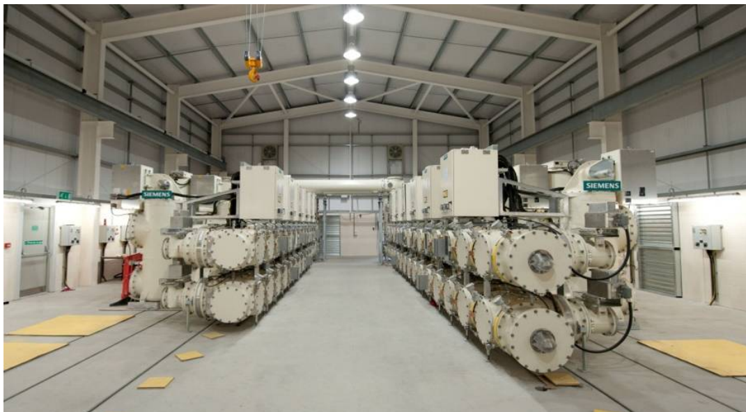
Figure 8 – Siemens 8DN8 GIS circuit breaker
