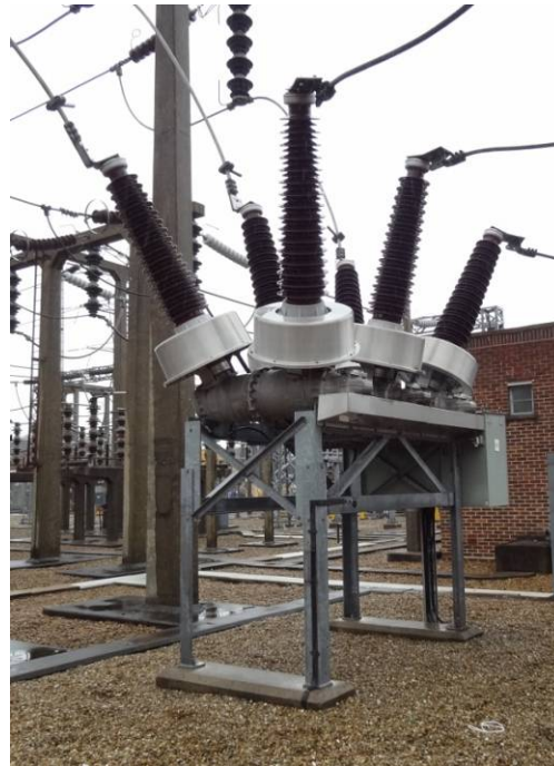
Figure 7 – Siemens 3AP1DT circuit breaker
