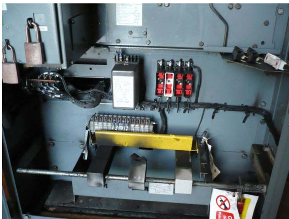
Figure 18 – Result of VT fuse failure for Reyrolle YMV
