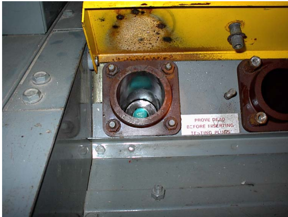
Figure 5 – Defective test bushing
