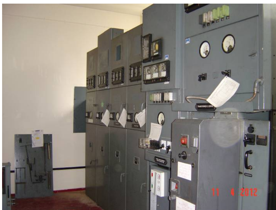
Figure 2 – Metropolitan Vickers type 'V1R' switchboard at West Green Primary
