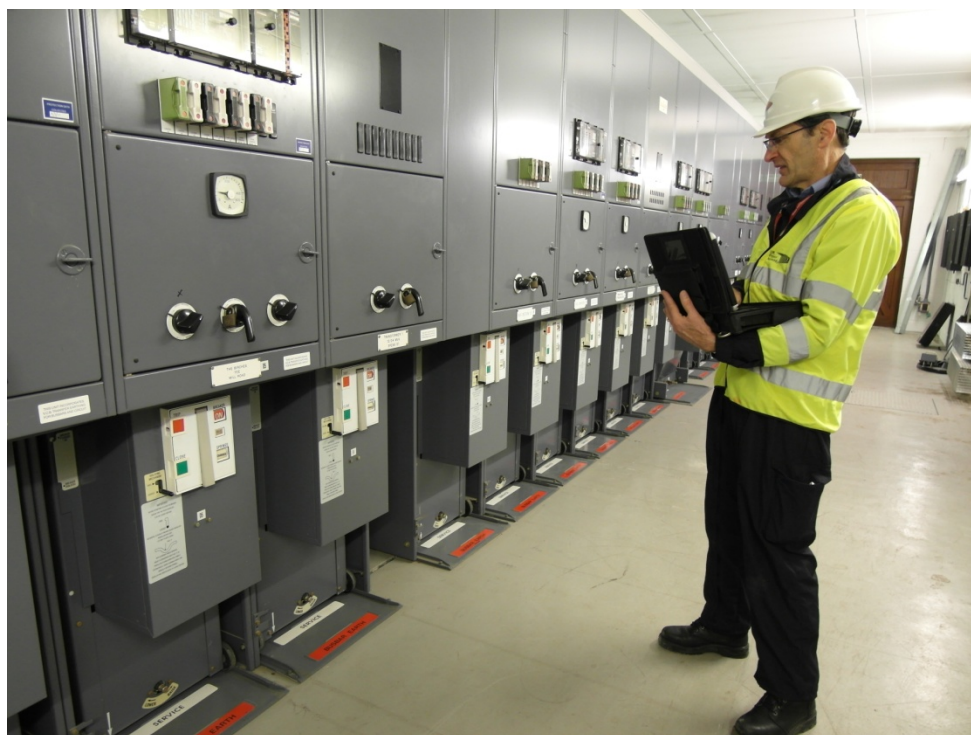
Figure 8 – Substation inspector with handheld device
