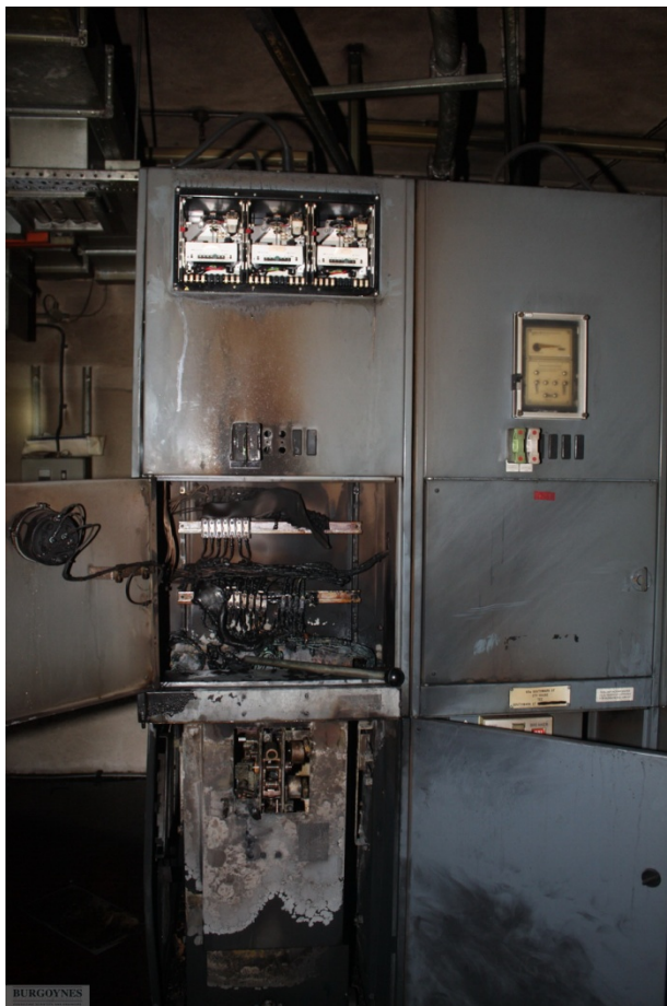
Figure 21 – GEC VMX: Failed 11kV panel
