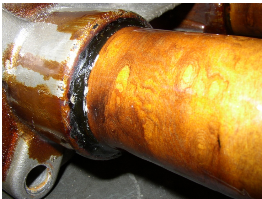
Figure 9 – Cable bushing in poor condition removed from AEI ‘QF’ switchgear at Hoddesdon Primary
